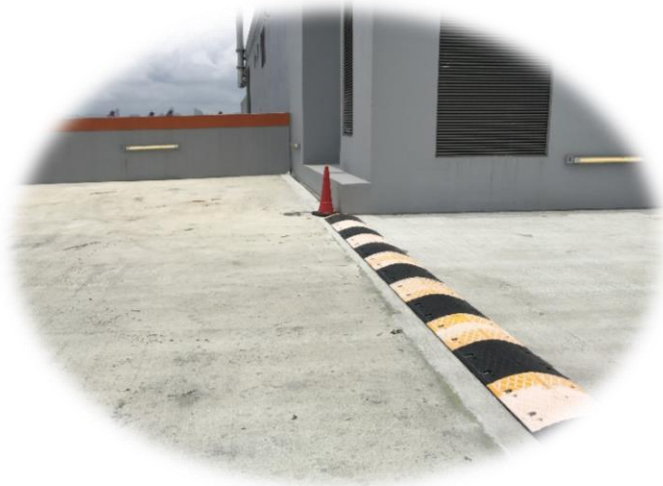
DRIVEWAY EXPANSION JOINT WATERPROOFING
